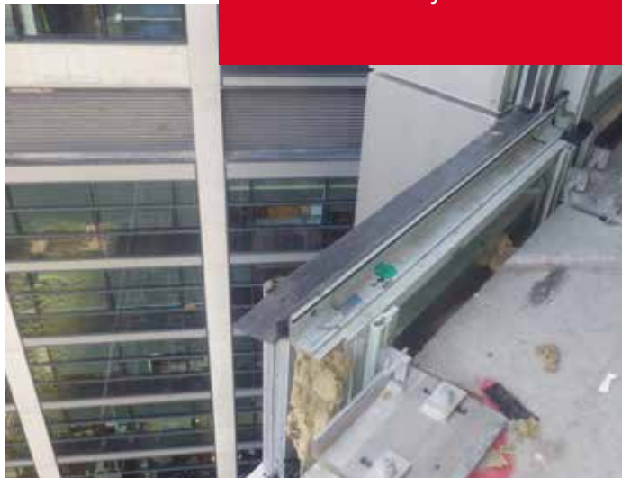
Stone wool insulation being installed as part of a curtain wall firestopping system
