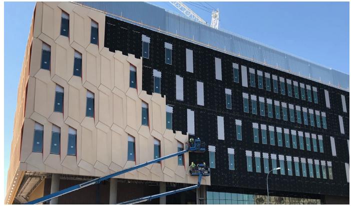
Figure 3: Exposed Cavityrock® Black during construction of Arizona State University in Tempe, AZ
