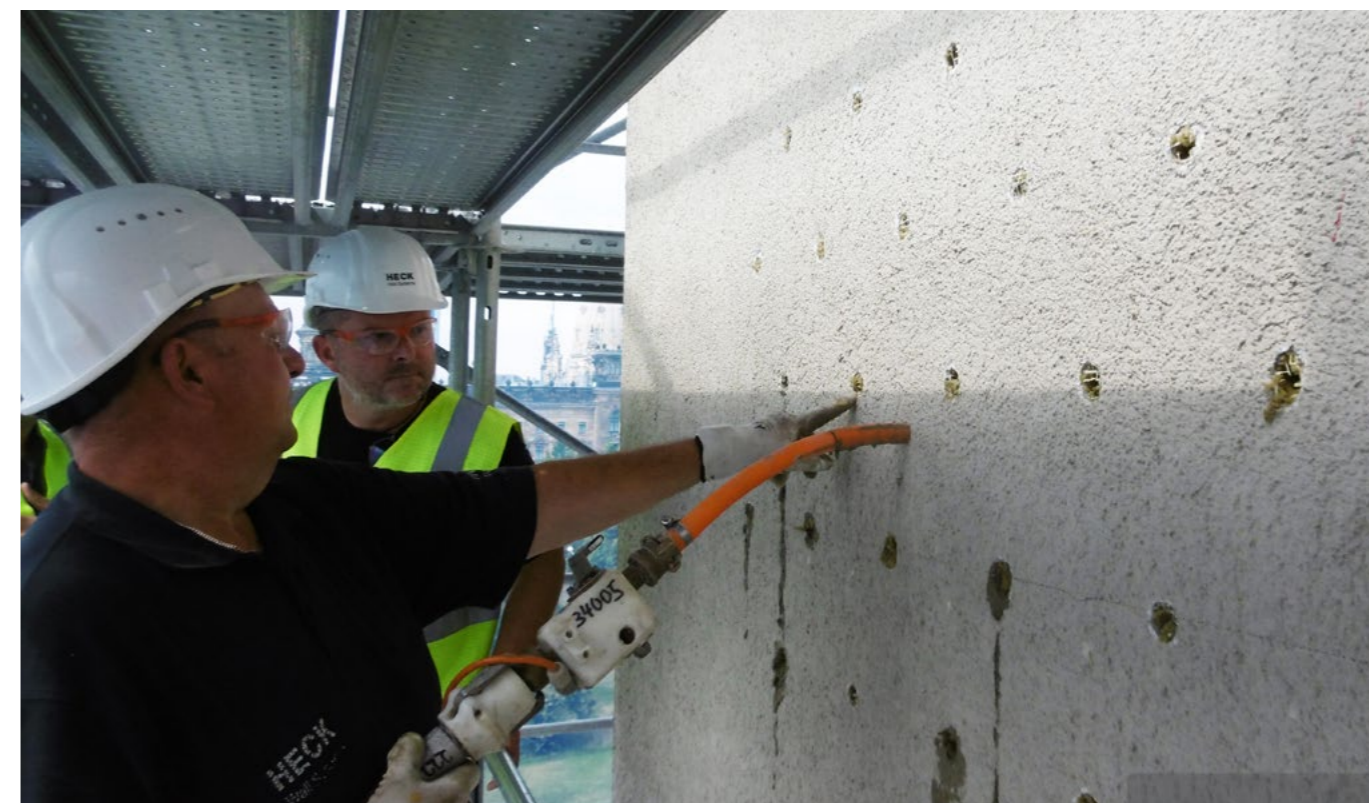
Before applying the ROCKWOOL external insulation, workers injected mortar behind the old mineral wool insulation layer across the facade.
