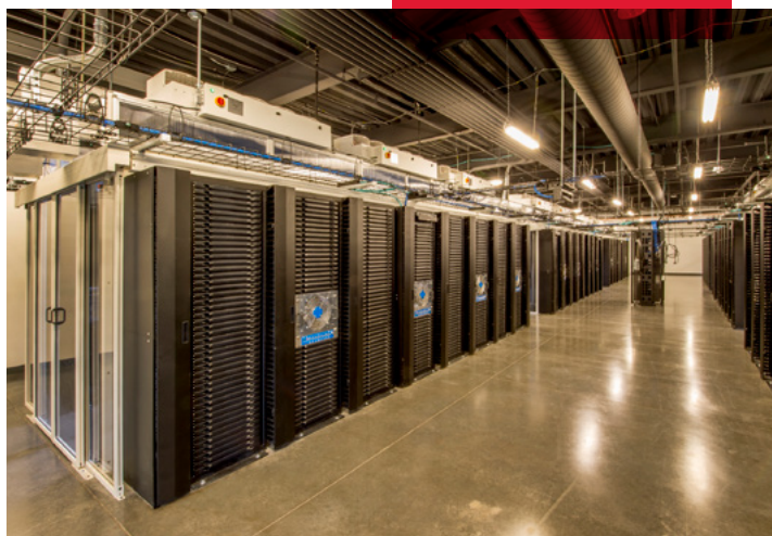
Figure 1: Interior of a modern data center with rows of high-density server racks.
