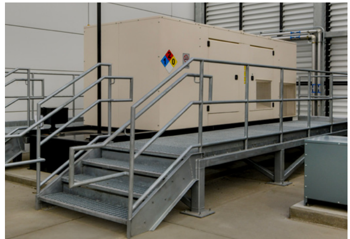
Figure 17: Diesel-fueled standby generator providing critical backup power for large-scale data center operations, equipped with an acoustic enclosure to minimize noise emissions.
