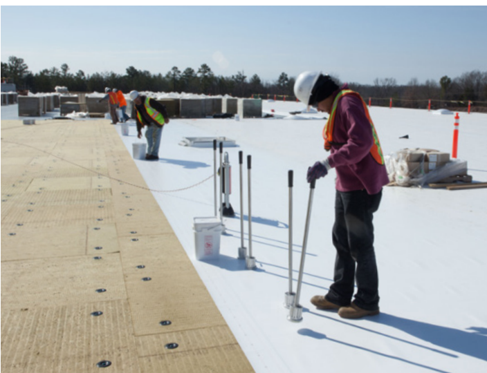
Figure 10: Installation of a PVC KEE single ply roofing membrane over ROCKWOOL Toprock® DD stone wool insulation.
