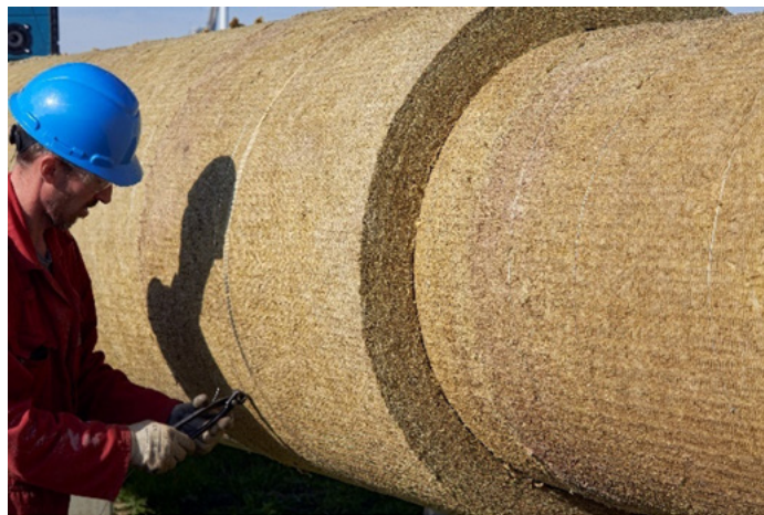
Figure 15: Installation of mandrel-wound pipe insulation on a high-temperature steam pipe, providing optimal thermal performance and personnel protection prior to metal jacketing.
